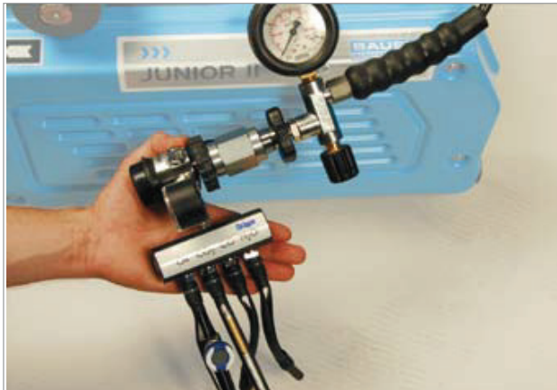
Measuring the air quality at the compressor
